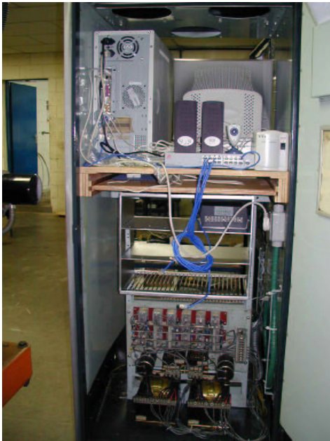
Fig. 14: Controller enclosure rear view.
