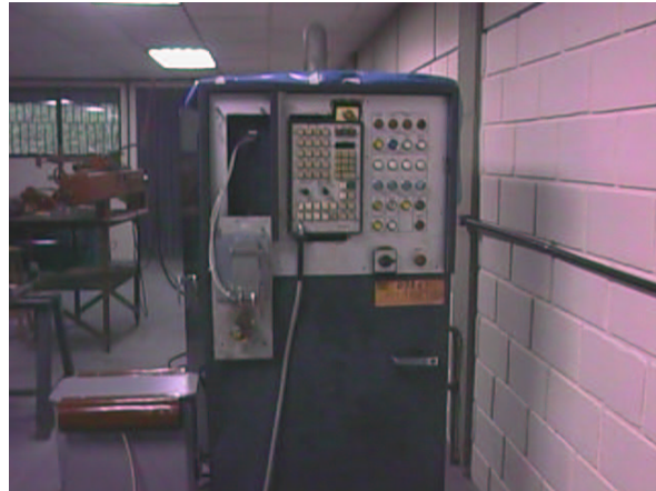
Fig. 6: Original ASEA IRB6 controller.
